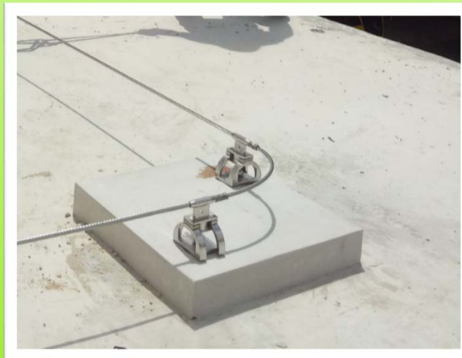
Figure 7: Curved Section on a Concrete Stump
